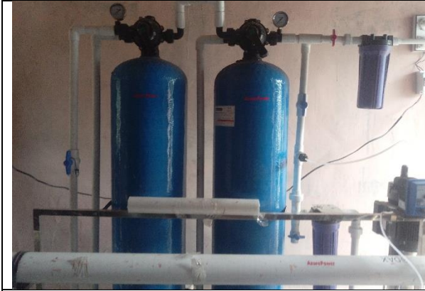
RO Water treatment plant at Kathoti School
